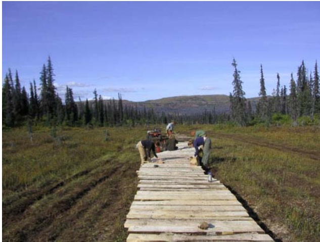
The District's Trail Crew and volunteers work to build this year's final section of boardwalk, approximately 1 mile south of Caribou Lake. The District will lay down the final boardwalk footage in 2005.
